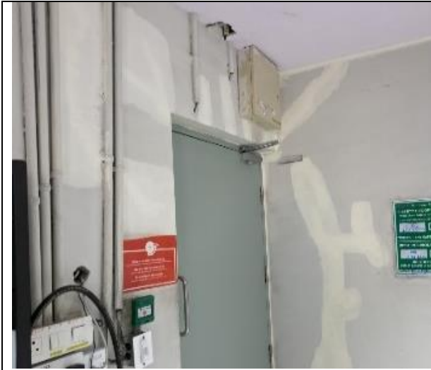
Major Cracks were observed in the SCR room which had been rectified.
