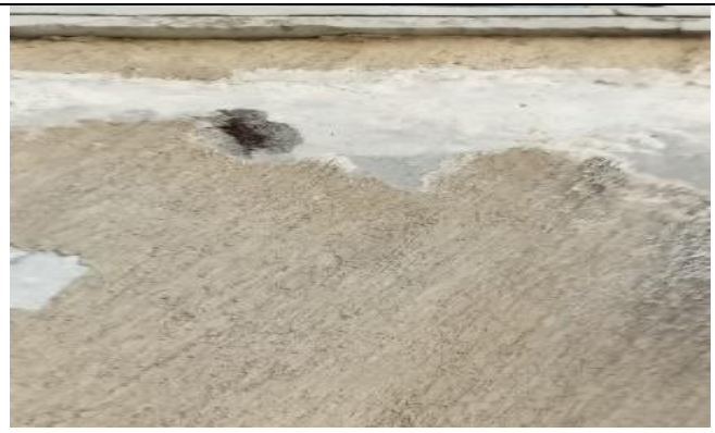
HYSD Steel Exposed near the staircase
