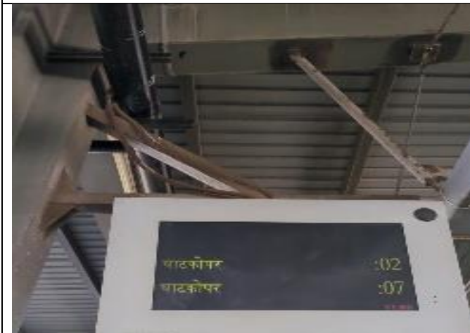
PEB Corrosion found at the platform level needed to be rectified.
