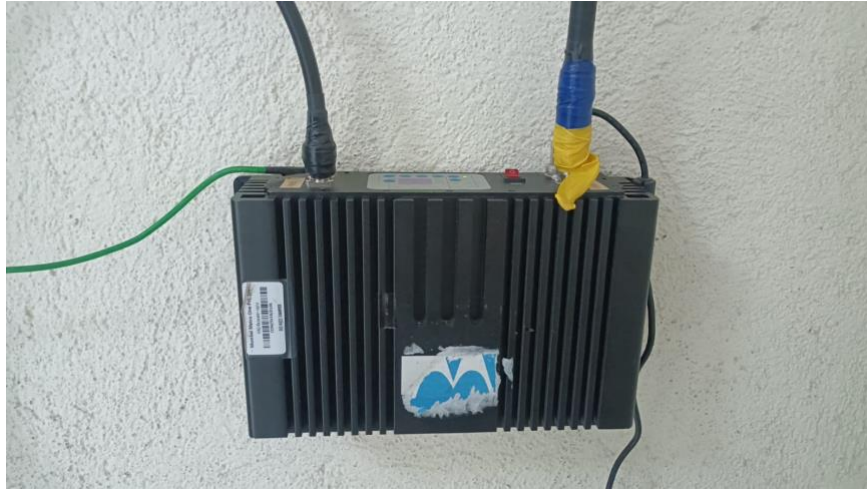
Radio repeaters at Azad Nagar & Versova is not functioning
