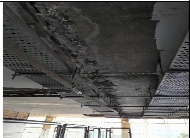
Unfinished work found at the concourse level needs to be rectified.
