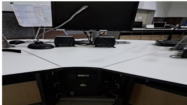
Radio CAD system is not functioning
