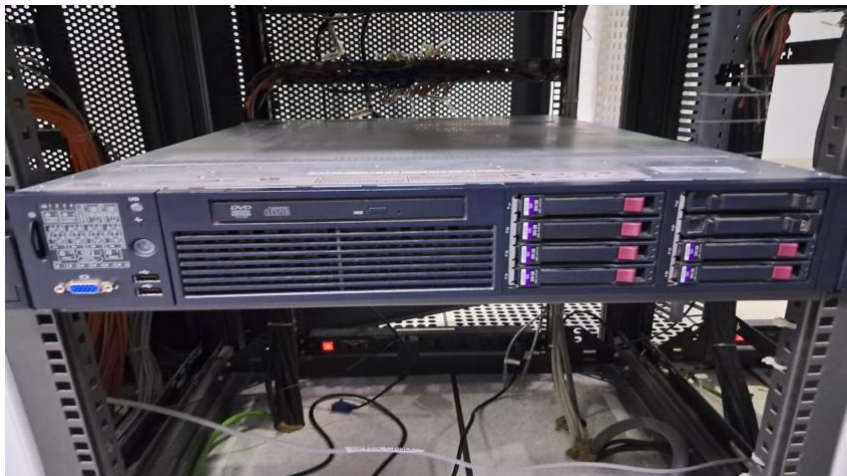
SDH NMS is not functioning
