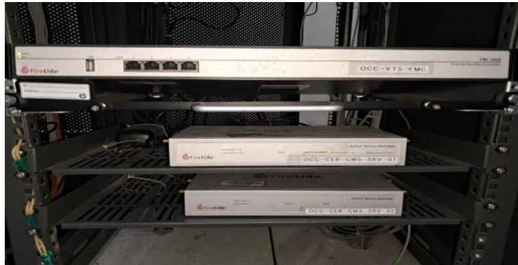
VTS-FMC 200 & Wireless Mesh Node is not functioning
