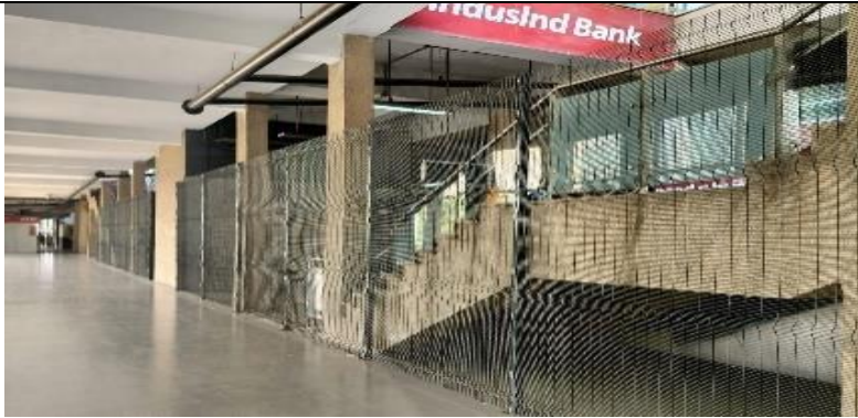
New Fencing had been provided at the Concourse level after the CMRS Inspection.
