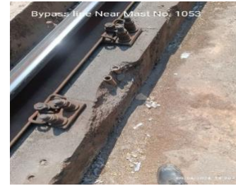
Plinth Beam in broken condition.
