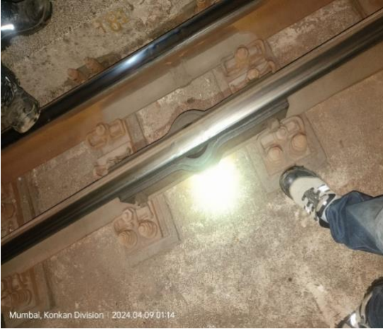
Weld protected with joggled fish plate
