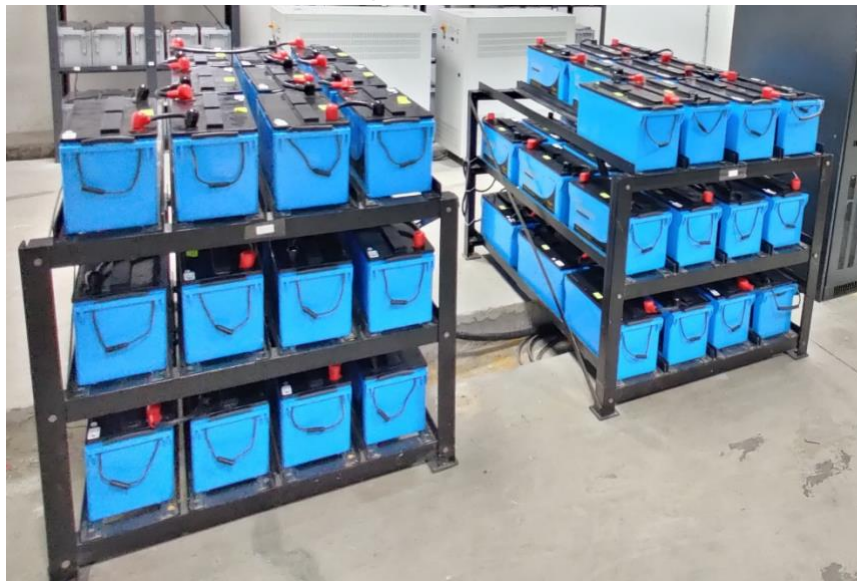
Newly installed Batteries
