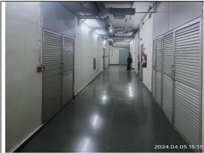
Corridor painting done by in-house team during CMRS but internal room paint need to be done
