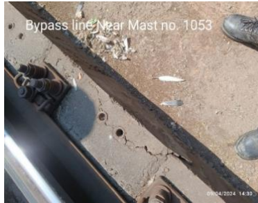
Plinth Beam in broken condition.
