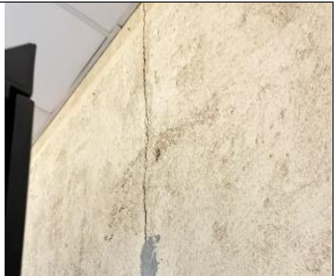
Cracks in the internal room wall had been observed which need to be rectified
