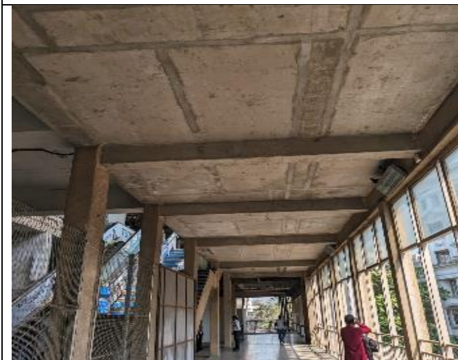
Concourse Level Passage finishing work not proper even construction joints are exposed.
