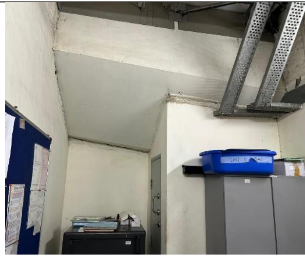
Major Expansion Crack at Audit Room / Revenue room between wall and Viaduct.
