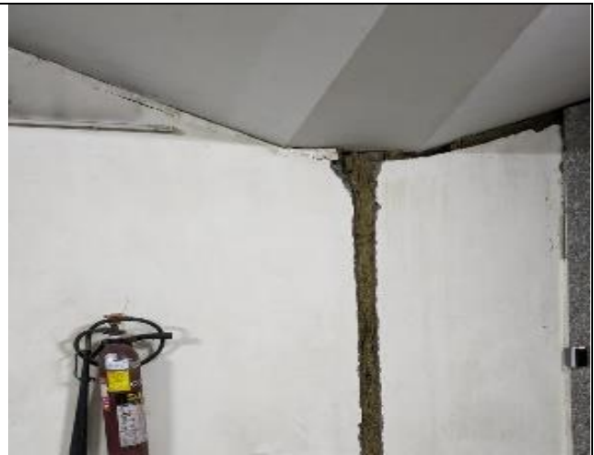
Major Gap Observed near Viaduct n bottom wall near passage observed
