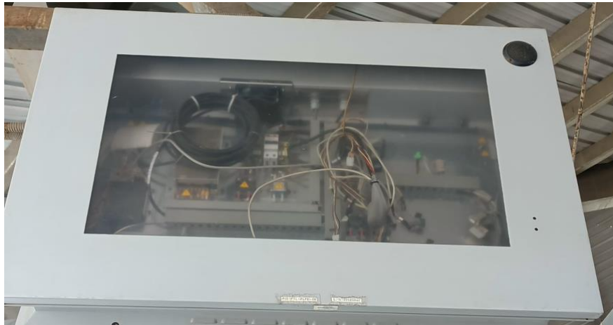
PIDS panel no -1 & 8 kept non-functioning
