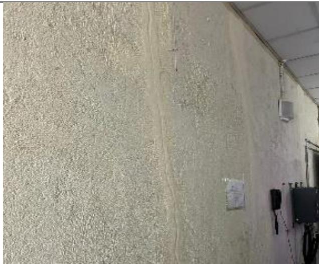
Cracks in the internal room wall had been observed which is need to be rectified.
