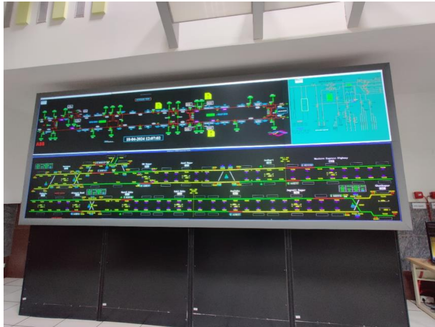
Newly installed RPS system
